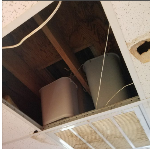
Roofing Leaks Inadequately Addressed
