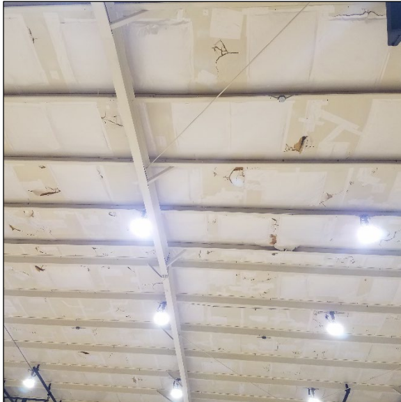
Gym Ceiling Deterioration
