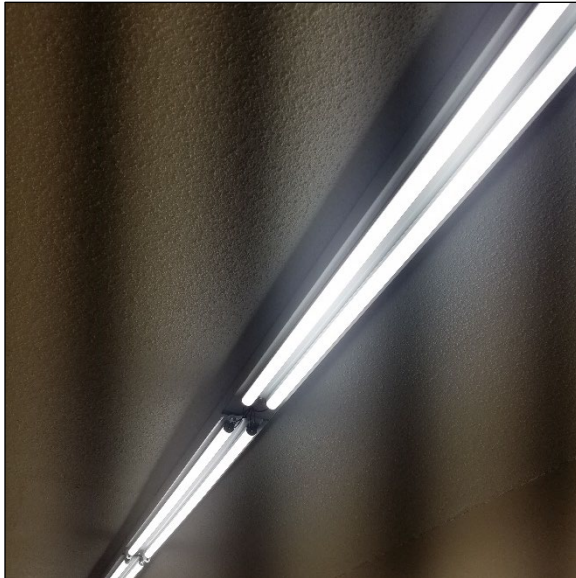
Uncovered Lighting Fixtures
