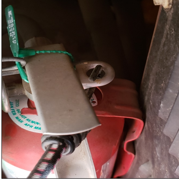
Trash Can Bungee Attached to Fire Extinguisher
